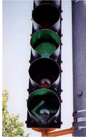
Traffic Signals (Gelcore)
